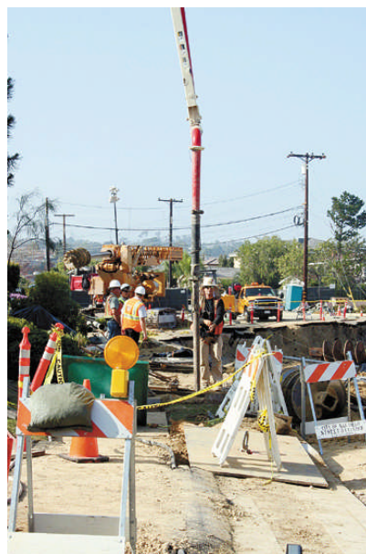
City workers cover holes where stabilizing pins were inserted with cement. The pins were put into place to keep the landslide from causing further damage. Photo by: Danielle Cadieux
